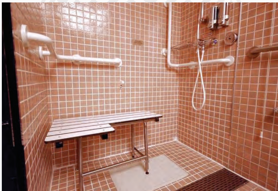
Figure 159: Accessible En-suite – Shower (Source : Cruise Critic.co.uk Cruise Reviews & News URL: http://cruiseforums.cruisecritic.com/showthread.php?t=984577 Accessed 20/08/09)
