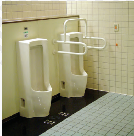
Figure 115: Urinal Showing a urinal with side and top grab bars, an emergency call button and detectable floor tactile tiles in front of the secondary urinal with hands-free flushing. Source: UDA & Associates
