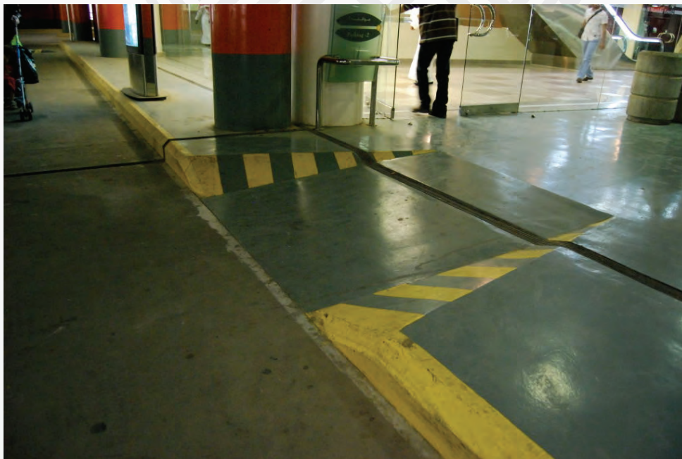
Figure 134: Example of curb-cut; note that the expansion joint makes access through this ramp difficult
